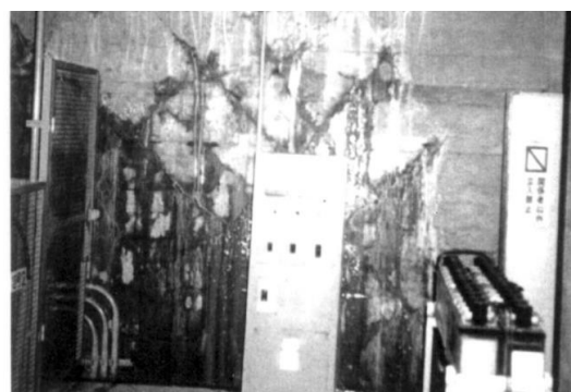
Photo 2 Cracks in the transverse wall in electric facility room.
