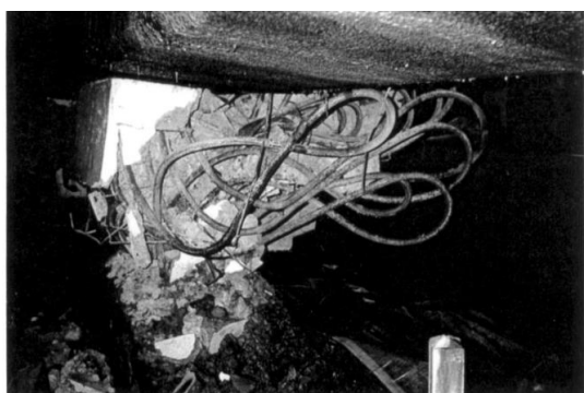
Photo 1 Collapse of no. 10 column in Zone A.
