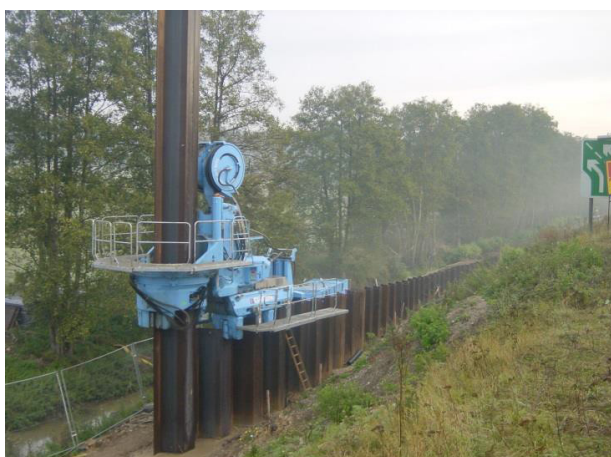
Figure 6: Installation & Filling Retaining Wall (in operation at the foot of sloping embankment)
