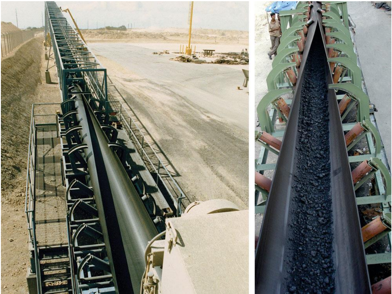
Figure 1. Tube belt conveyors
