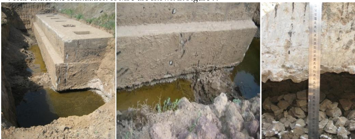
Figure 9. Voids underneath the bottom of the MF#3 foundation
