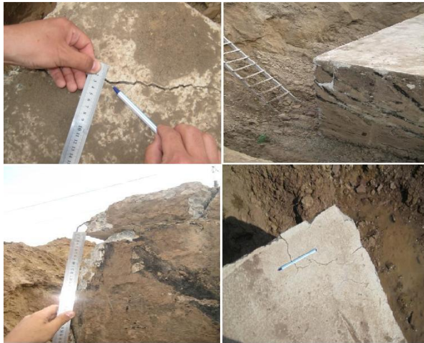
Figure 5. Chips and potholes found on foundations
