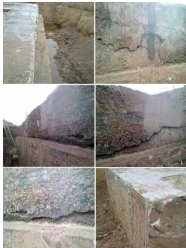
Figure 6. Detected defects in foundation structures
