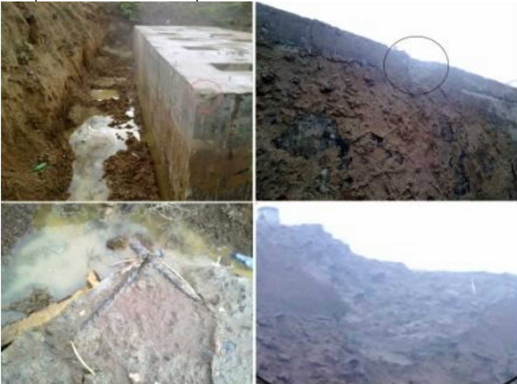
Figure 4. Failure of concrete foundations
