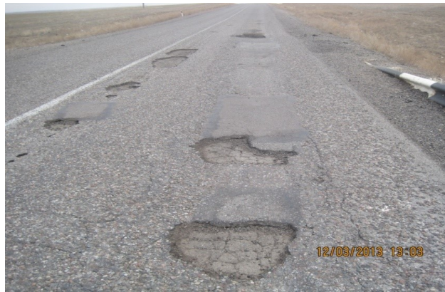
FIGURE 1 – Example of deformation regarding to frost heaving and thawing
