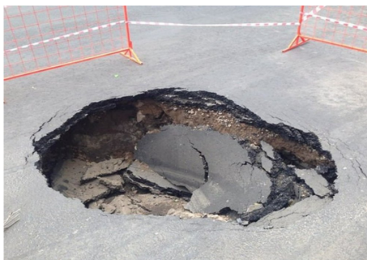
FIGURE 2 – Another example of deformation regarding to frost heaving and thawing
