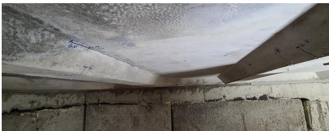
Figure 10. Cracks in floor slab and floor slab ribs
