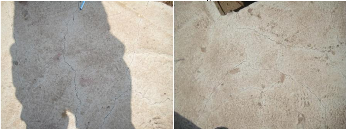
Figure 8. Cracks in the surface of the MF#4 foundation
