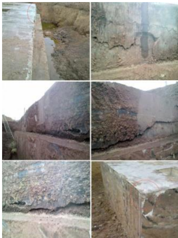
Figure 6. Detected defects in foundation structures
