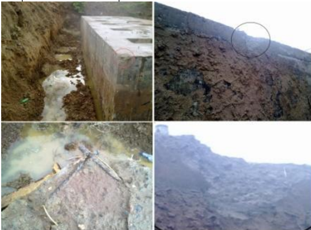
Figure 4. Failure of concrete foundations
