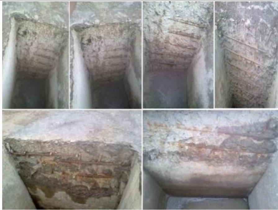
Figure 7. Corrosion of fittings in foundation wells for props
