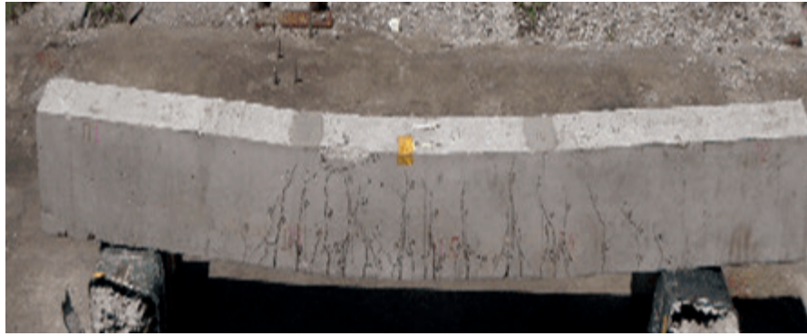
Figure 5. Failure of a reinforced concrete beam without reinforcement
