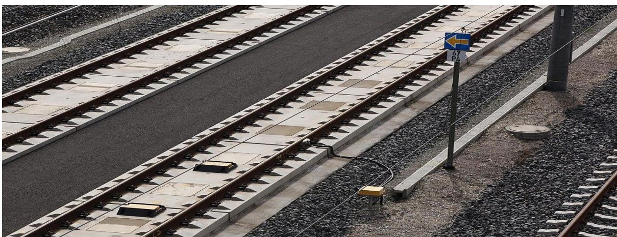
Figure 1 ETCS floor devices: eurobalises (between rails) and wheelset counting device (fixed on rail), Erfurt — Leipzig line, Germany
