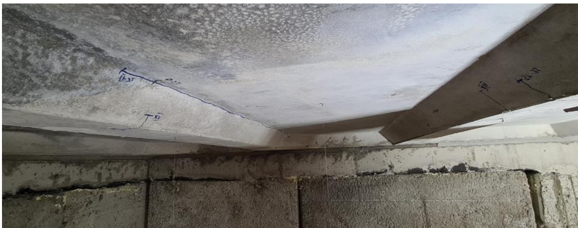
Figure 10. Cracks in floor slab and floor slab ribs
